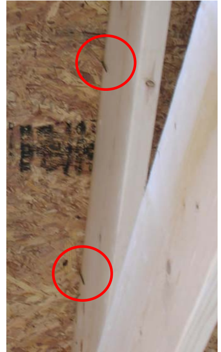
Picture of nails missing the truss
