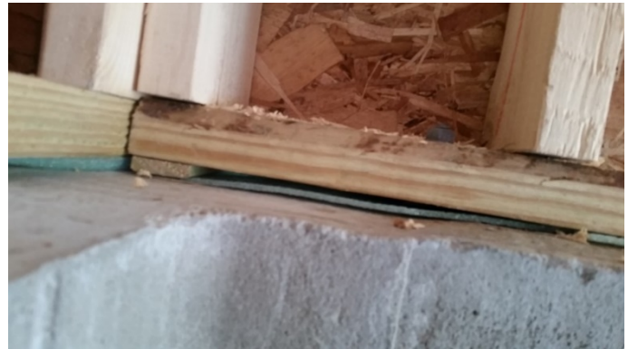
Figure 1: Flexible foam gasket installed to help reduce air infiltration between concrete foundation and sill plate. Notice the gaps and lack of air sealing.
