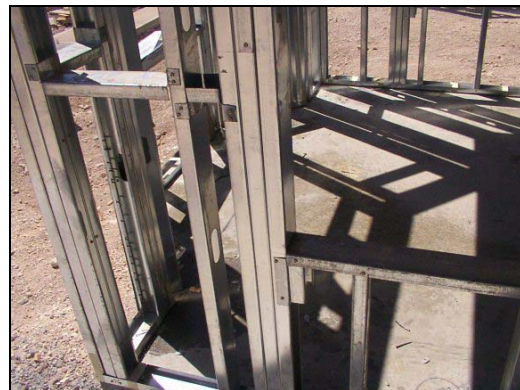
Wall section in home under construction. The short piece under the window opening connects the bottom of the window framing to the adjacent studs and is prefabricated "off-line" at the panel facility.
