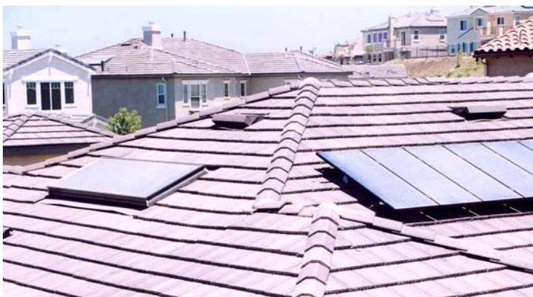
Figure 4 – Low profile solar pre-heat of domestic water (on left of roof) at PATH field evaluation in San Diego (source: Toolbase)
