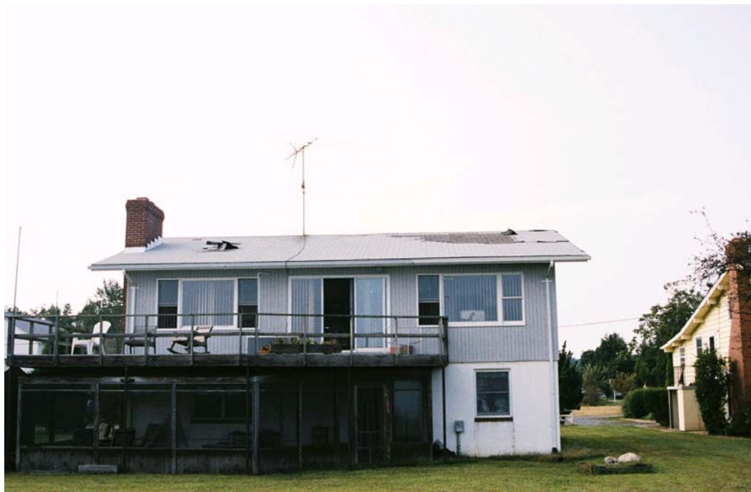
Figure 2 - Roof covering damage on Maryland home from Hurricane Isabel in 2003 (provided by Jay Crandell of ARES).
